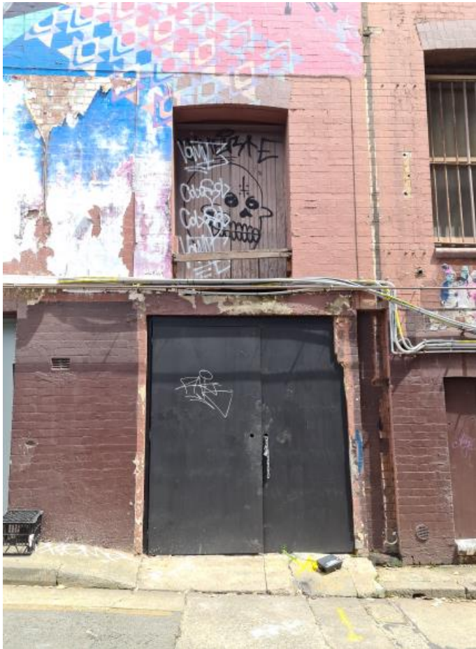
Figure 49: Existing door opening along Foley Street, originally approved as location of loading dock
